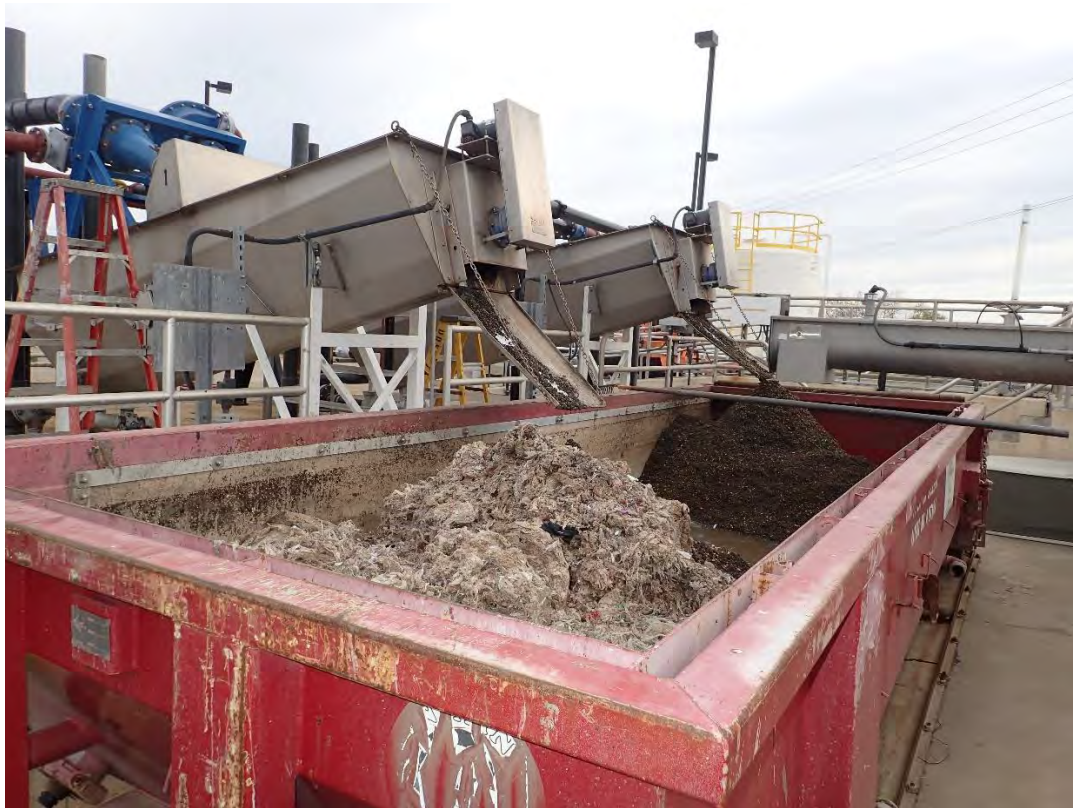
4. Waste from screening and grit removal.
