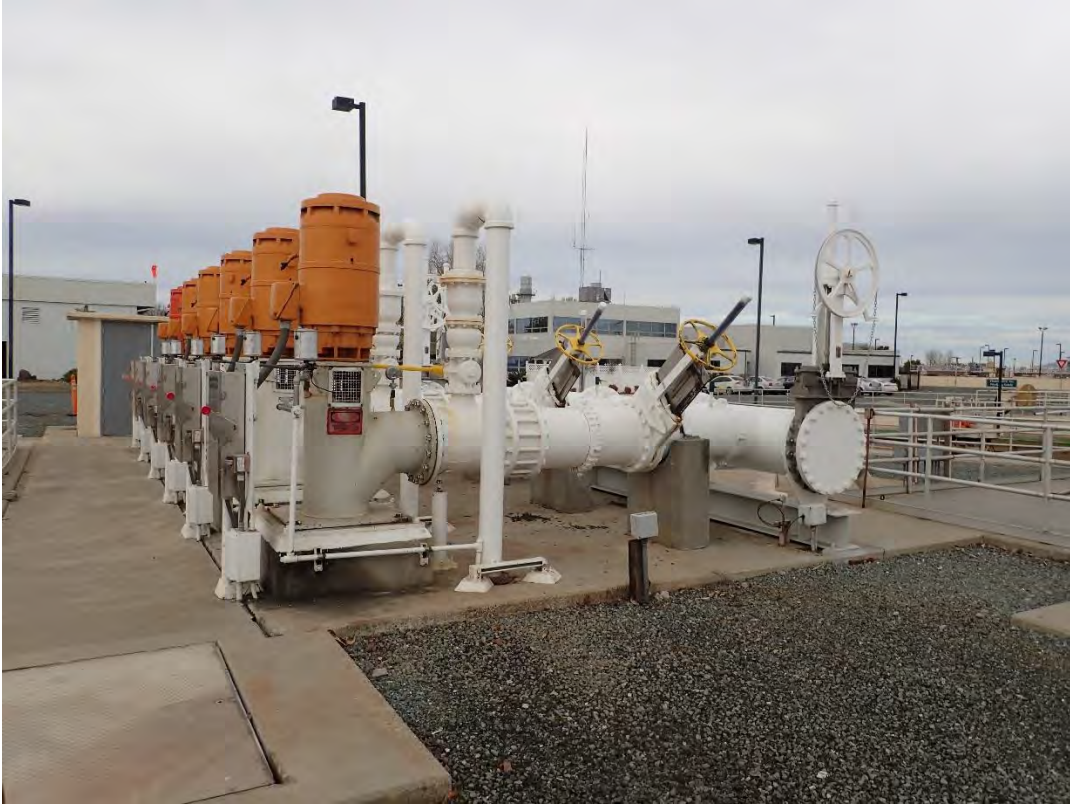
5. New pumps. They were formerly in sump during the last inspection.
