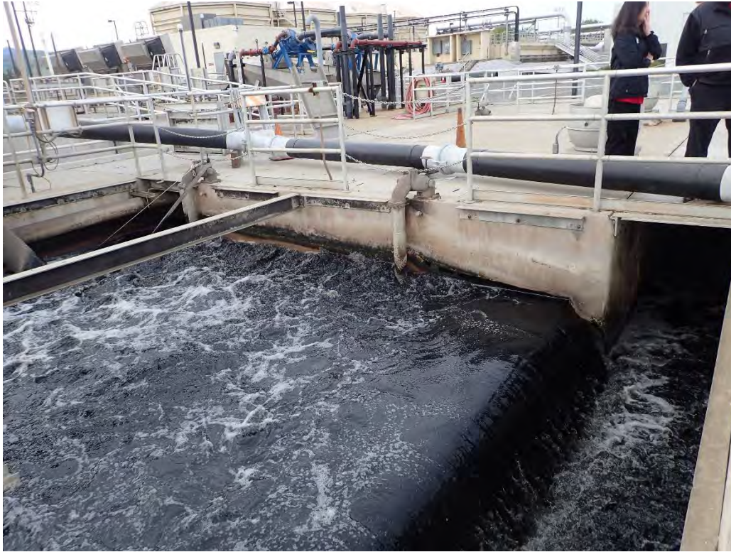
3. Grit removal chamber.
