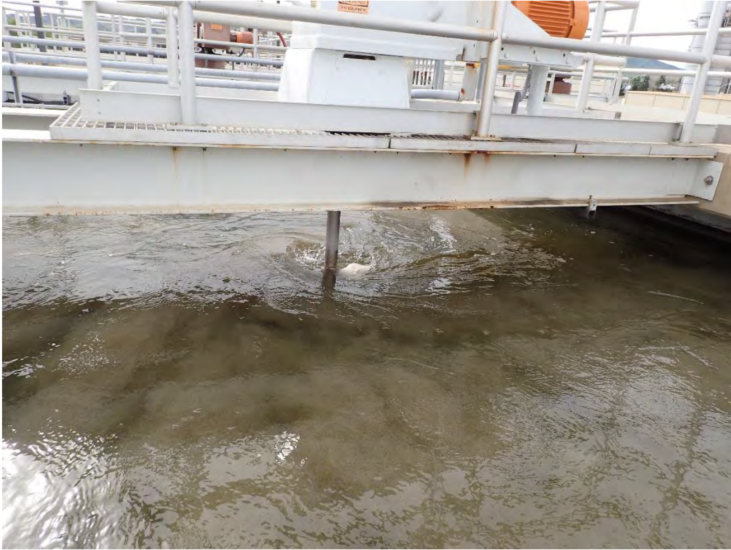
13. Flocculation tank at recycled water plant.
