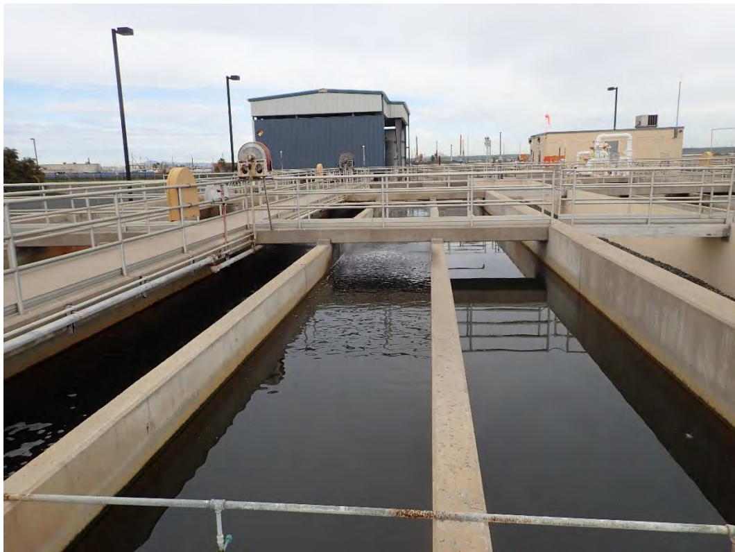
10. Chlorine contact chamber.
