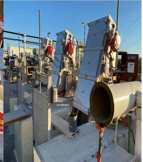
New bar screens
