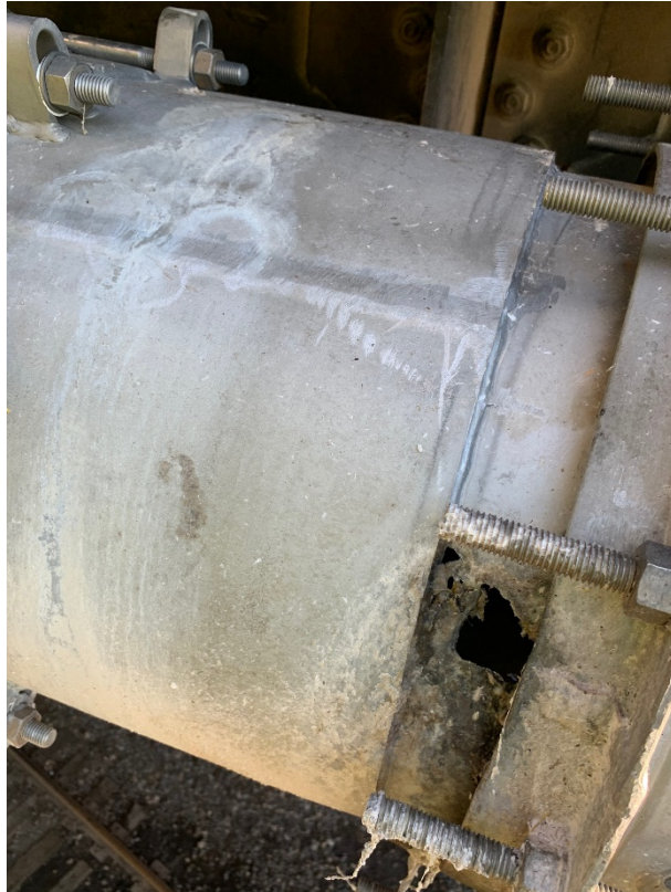
Corrosion failure at flowline of expansion joint
