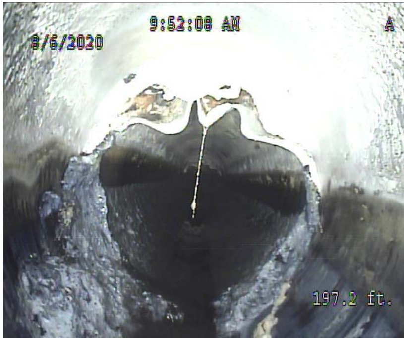
PE liner delamination at pipe joint (restricts flow capacity)
