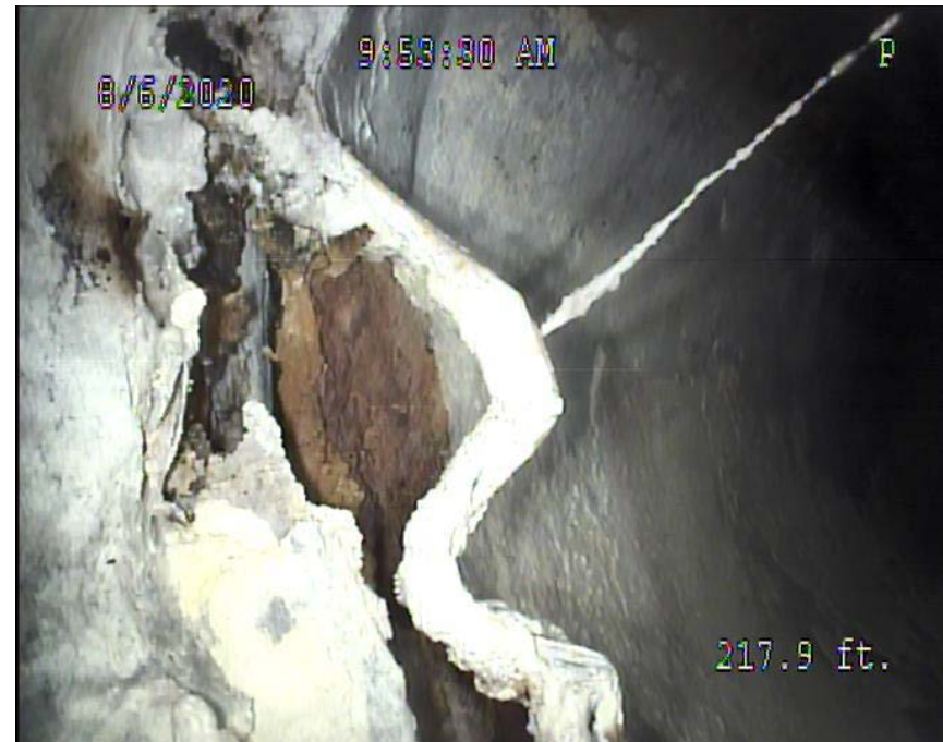
Ductile iron pipe corrosion at PE liner failure
